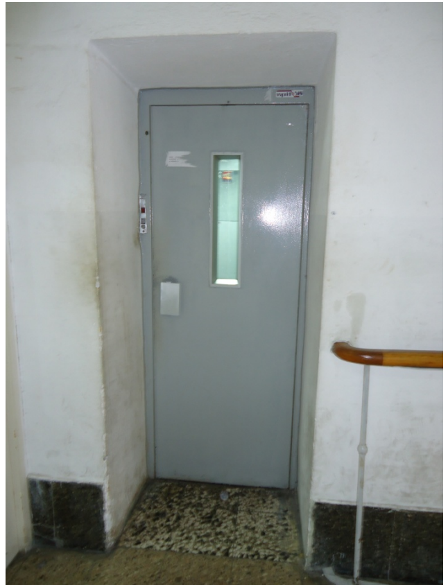
Picture 9 : Main elevator
